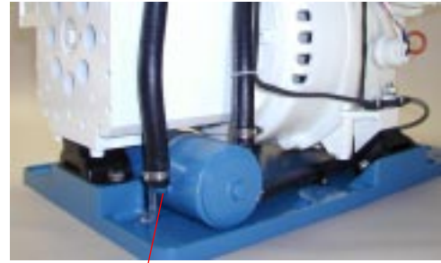
Heat Exchanger Outlet
