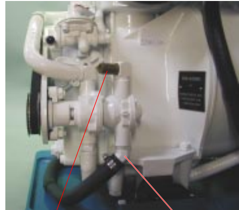
Raw Water Inlet
